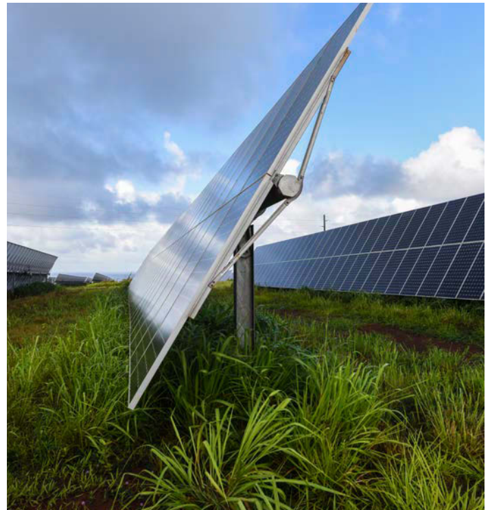
AES Lawai Solar Project- Kauai. Photo by Dennis Schroeder, NREL 58006
